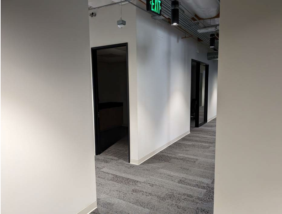
17. View of the interior of Unit C-200 showing non-asbestos sheetrock and joint compound.
