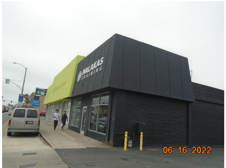
Existing north building elevation facing driveway to be updated with new materials and paint
