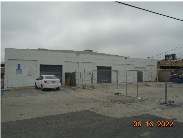
Existing rear of the building and condition of the rear surface parking lot to be reconfigured and restriped to comply with parking design standards
