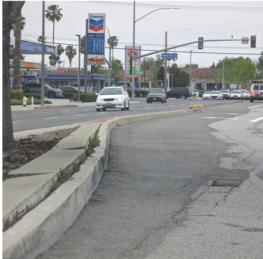
More buckling concrete
