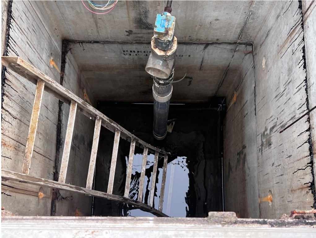
Figure 2-17: Water Level Sensor Vault
