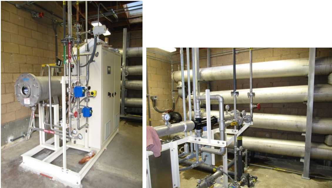
Photographs 1 and 2: Ozone Generator and Ozone Injection/Contacting System
