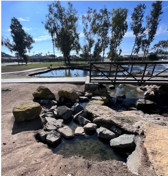
a) Major Crack and Leak Shoreline
