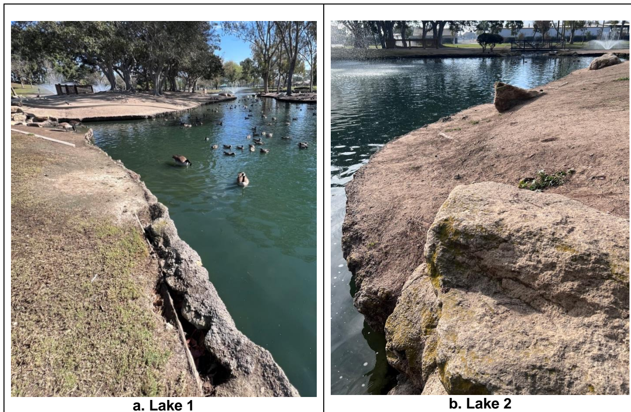
Figure 2-9: Erosion at Lake Shorelines
