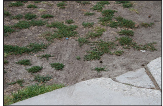
Damaged sidewalk in need of repair.
