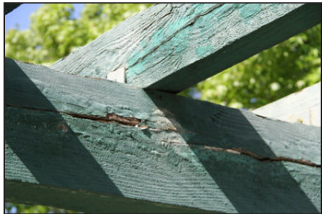
Shade structure members in need of repair.
