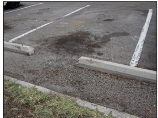
Asphalt parking stalls in need of repair and resurfacing.
