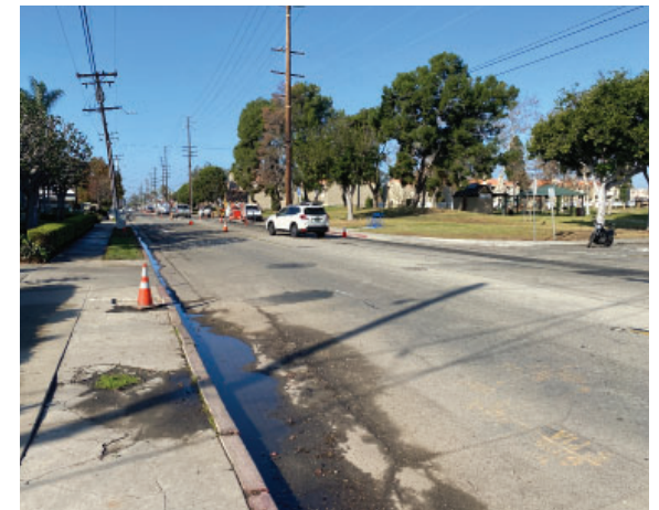
Cracked and buckled sidewalks near Wilson Park
