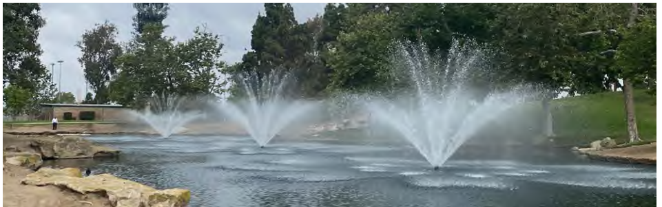
The existing six fountain spray systems are popular features activated on a timer and push water onto the shore during minor wind events.
