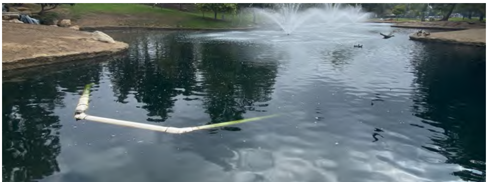
The Existing PVC recirculation piping is not properly secured to the bottom of the lake and requires replacement.
