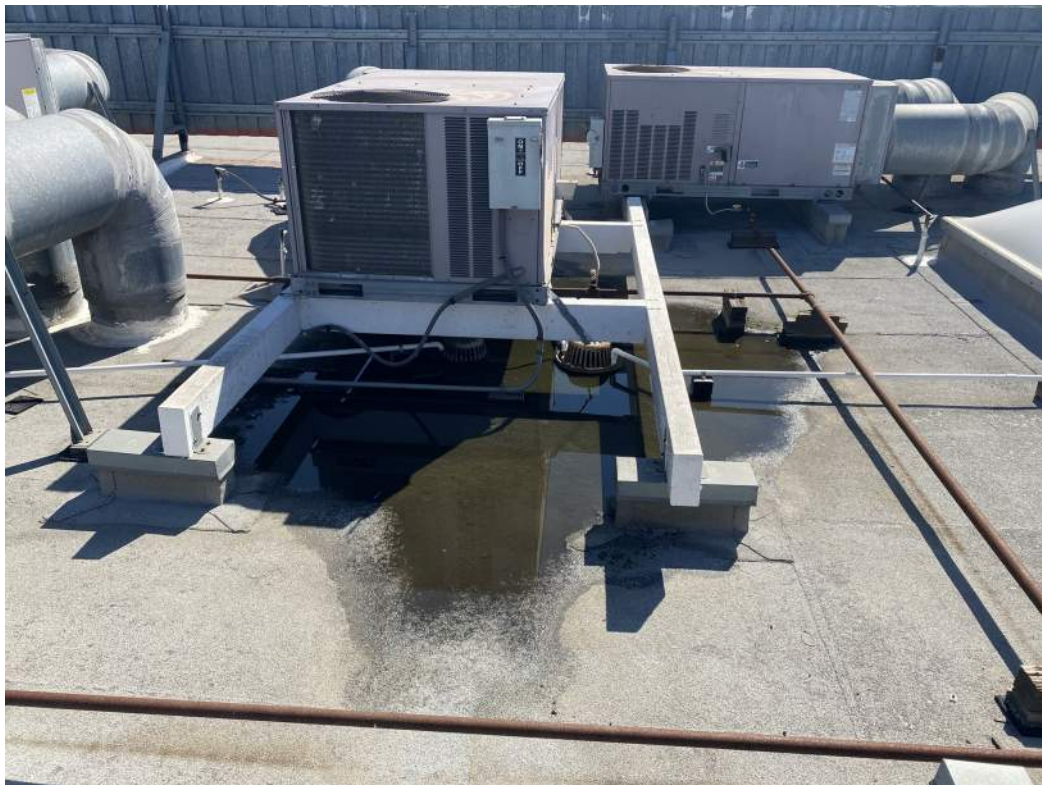
FIG 8: PONDING AT EXISTING ROOF DRAIN. CONDENSATE LINE CAN BE SEEN FROM LEFT EXACERBATING PONDING ISSUE.
