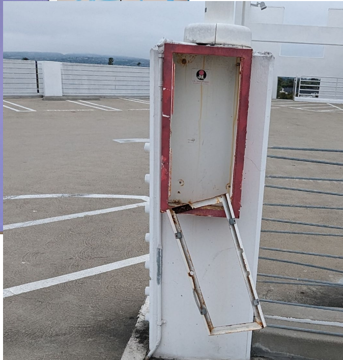
Fire Extinguisher Missing
