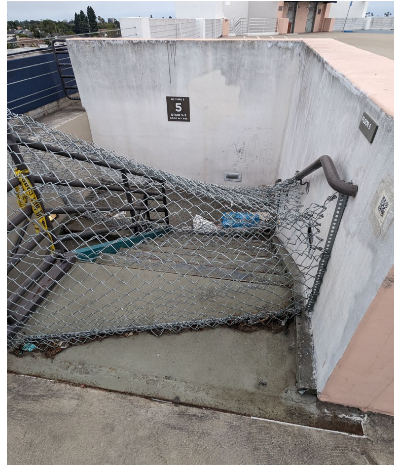
Stairway Blocked by Chainlink Fence
