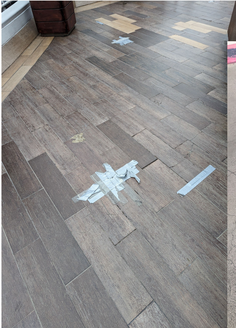
Duct Taped Tiles
