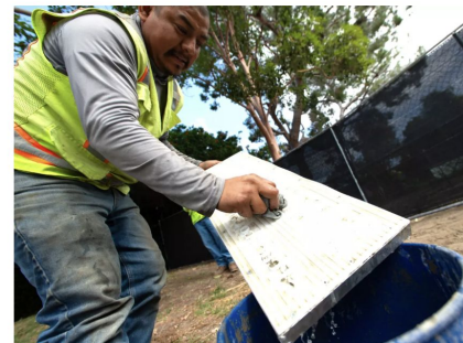
Marco Reyes cleans a mold to press poems into a concrete path leading to a new playground at Brentwood Park in Costa Mesa. (Eric Licas)
