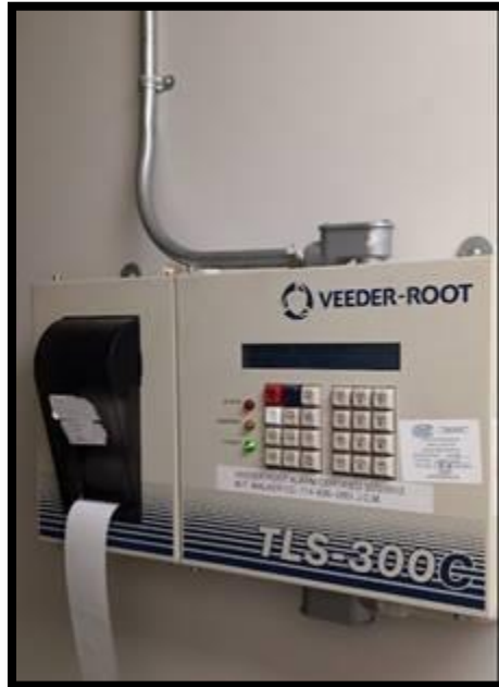
Figure A1.1.1 - As part of the base bid Contractor shall disconnect and remove the Veeder Root Box in the Police Department basement. Existing low power shall be capped in a covered electrical box.
